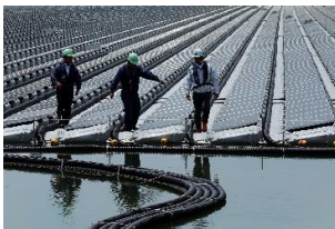
Figure 31: Floating solar installation in Japan
